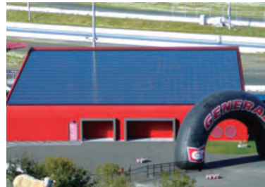
Solar panels installed at the Infineon Raceway
